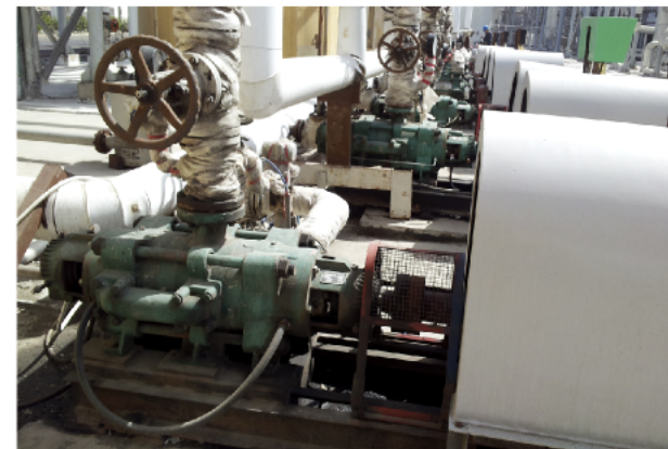
平煤集团联碱厂母液泵应用现场（型号：ZDF150-30×7 数量：7台套）Pingmei Group Al factory Mother liquor pump working site (Model: ZDF150-30X7, 7sets.)
