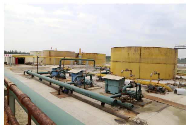
中盐集团采卤泵、输卤泵应用现场（型号：DF280-65×10 数量：6台套）China National Salt Industry Company brine extraction pump working site (Model : DF280-65X10, 6 sets)
