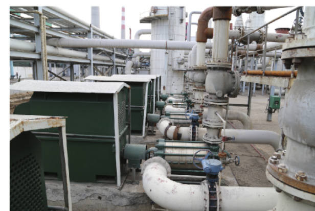
山东魏桥集团不锈钢多级泵应用现场（型号：DF450-60×7 数量：7台套）Shandong weiqiao Group Stainless Steel Pump Working Site (Model : DF450-60X7, 7 sets)
