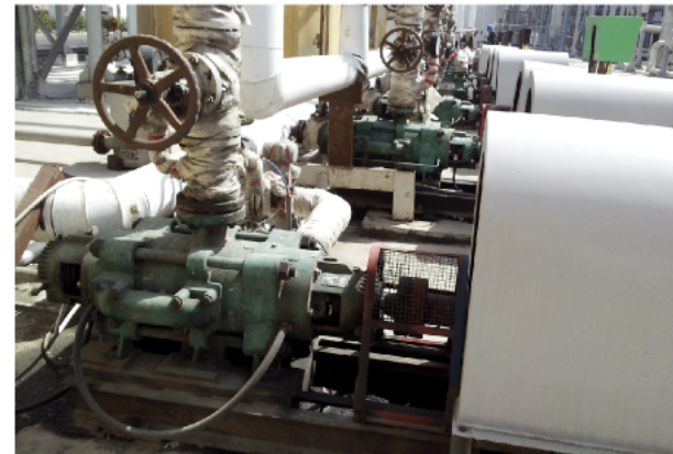
平煤集团联碱厂母液泵应用现场（型号：ZDF150-30×7 数量：7台套）Pingmei Group AI factory Mother liquor pump working site (Model: ZDF150-30X7, 7sets.)
